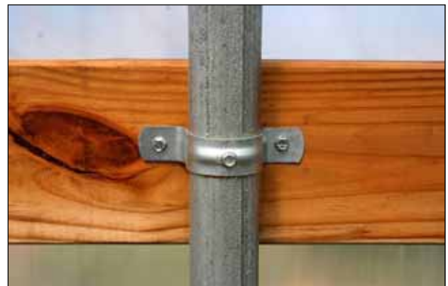
Figure 16. Peak-style high tunnel framing - side view showing close up of batten board fastening.
