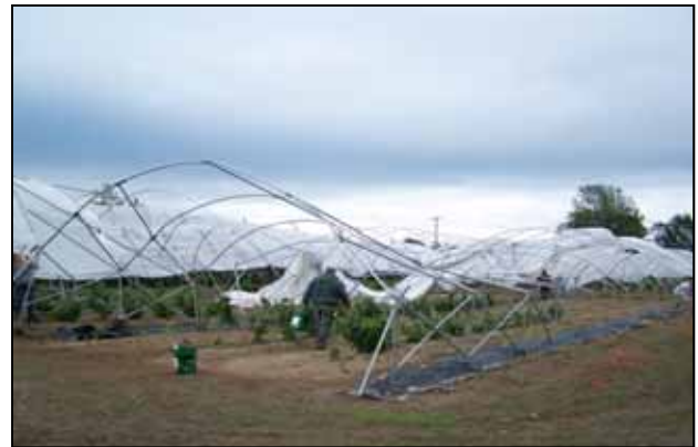
Figure 14. High wind damage to a multi-bay style high tunnel as remnants of Hurricane Ike passed through Upstate New York, fall 2008.
