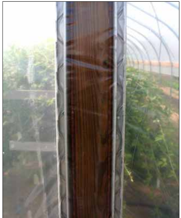
Figure 26a. Fastening the plastic to batten boards with wiggle wire. The wire secures the plastic by pinching it in a channel.
