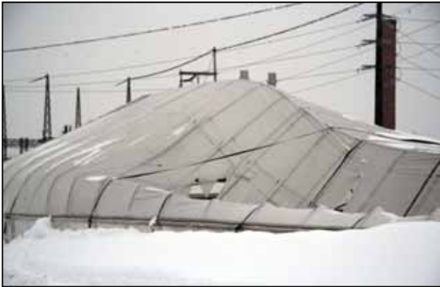
Figure 13a. Peak-style high tunnel collapsed under heavy snow load, February 2010, Ithaca, NY.
