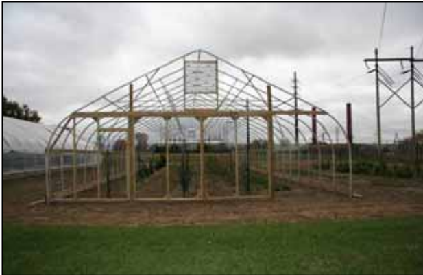
Figure 17. Peak-style high tunnel framing - front view shows end framing. Doors open outwards at both ends.
