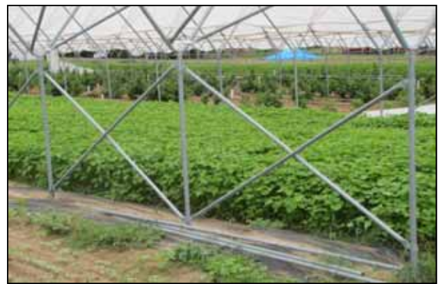
Figure 24. Diagonal pipe and wire braces.
