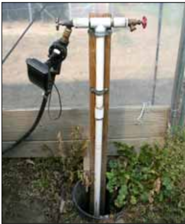
Figure 9. Drip irrigation ingress pipe with in-line water filter and faucet for hose attachment.
