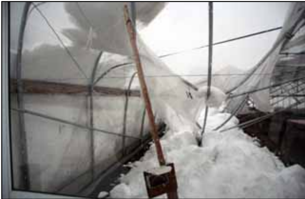
Figure 13b. View inside collapsed tunnel, February 2010, Ithaca, NY.
