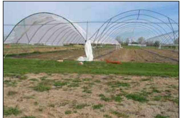
Figure 28. Bundles of plastic are placed in the troughs between bays then pushed to the peak, unfolded, and secured in place with ropes (left).
