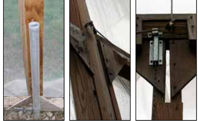
Figure 19. End door construction (L to R) door stop, pulley system for door closure, door closure.
