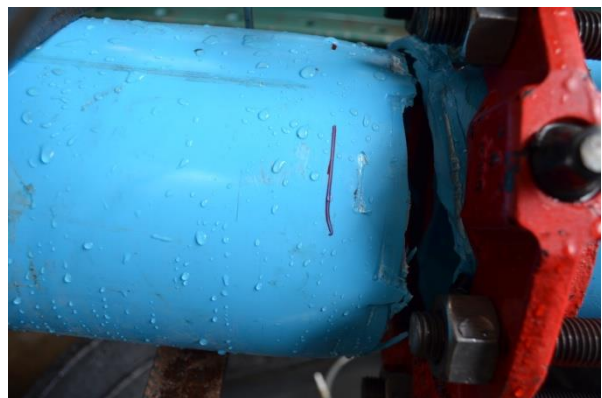
Figure 4.16. Joint Tension T2 – Close Up of Ruptured Pipe
