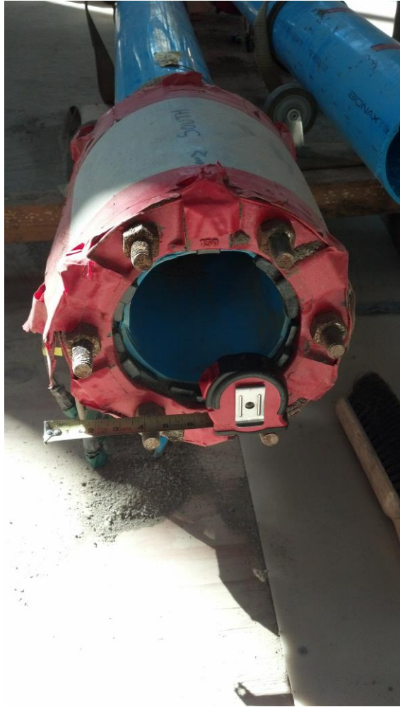
Figure B.7. South Joint Showing Ruptured Pipe and Joint Protective Enclosure
