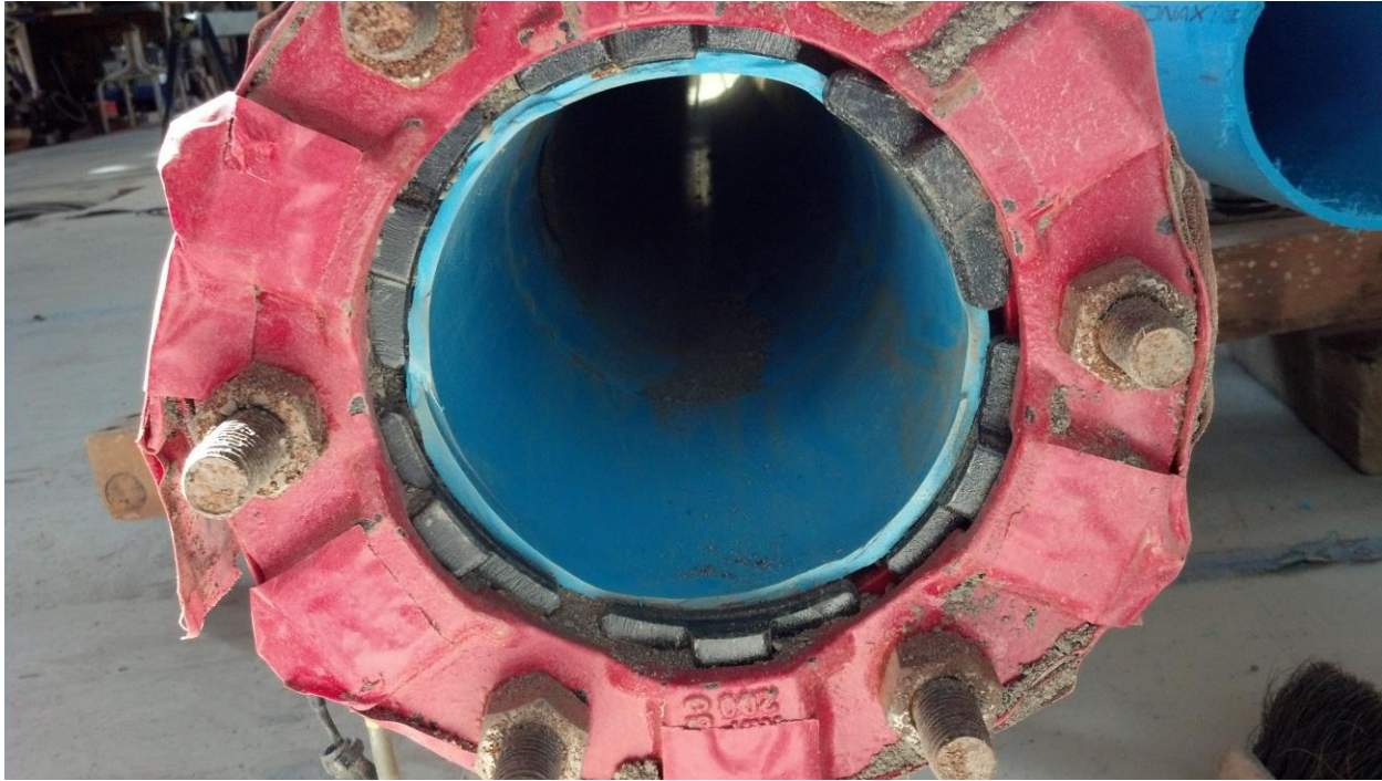
Figure B.8. South Joint Showing Ruptured Pipe
