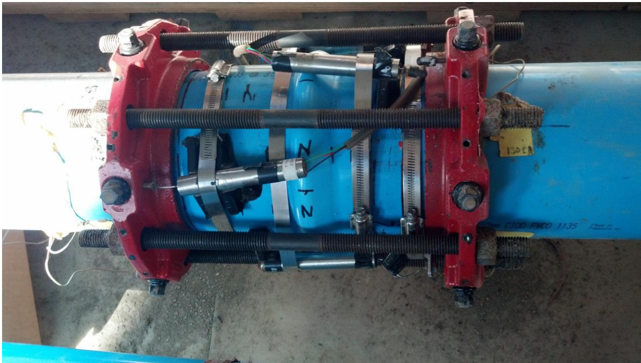
Figure B.9. North Joint after Test with Protective Enclosure Removed
