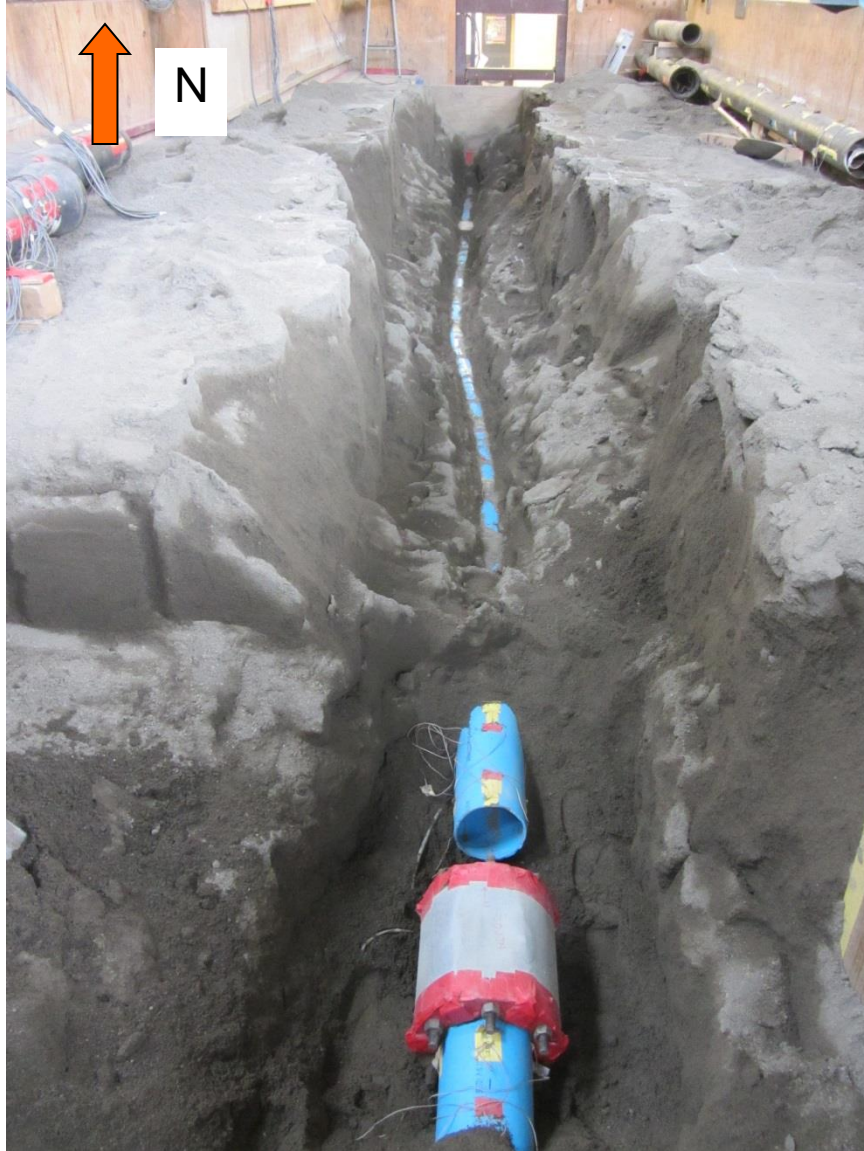
Figure B.4. South Joint after Pipe Rupture
