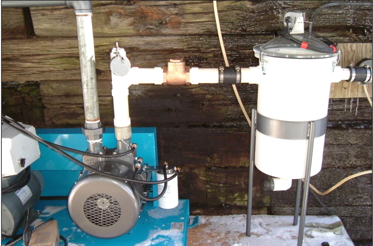
Vacuum pump and moisture trap set up outside the sugarhouse at the Arnot Forest
