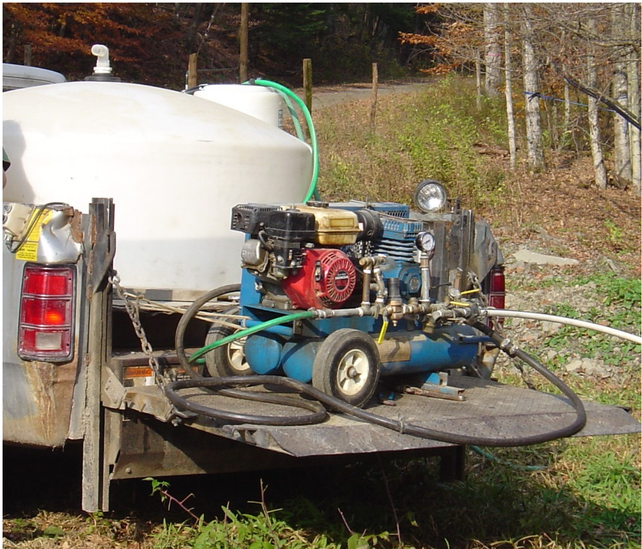
Pickup truck with water tank, air compressor and water pump set up to rinse mainlines.
