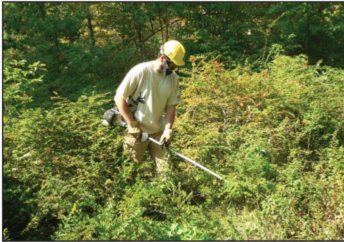
A brush saw, including personal protective equipment, is an example of a organic, mechanical approach to controlling competing vegetation near planted seedlings. Photo – J. Ward
