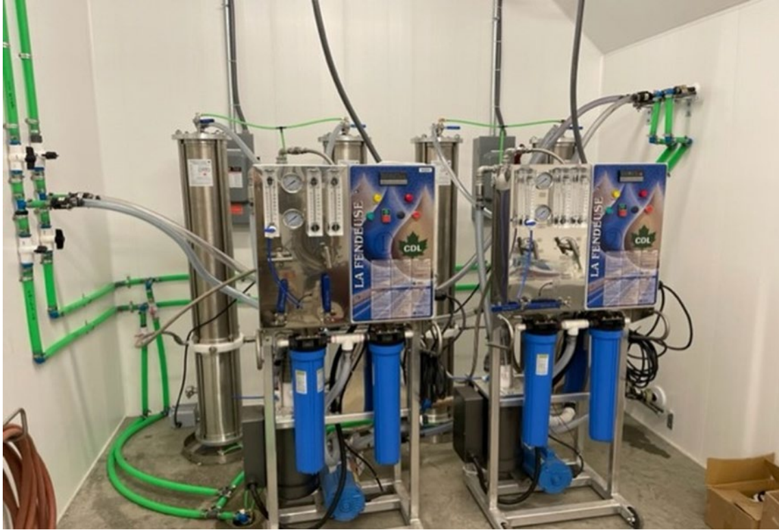
Energy saving reverse osmosis units at Arnot Maple Lab
